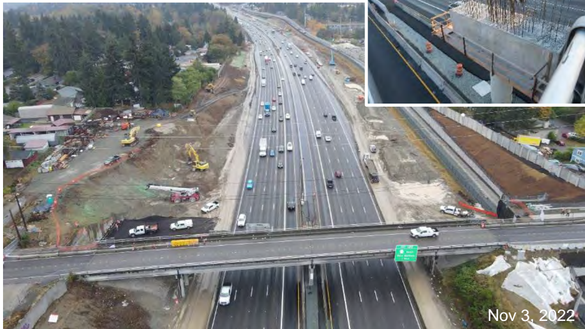
SR 509 work zone showing progress on the new South 216 th Street Bridge
