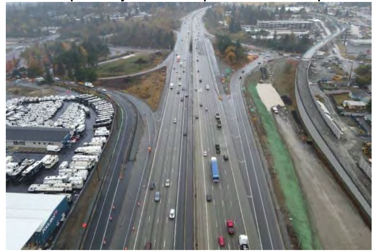
Widening I-5 near the SR 516 interchange to support the SR 509 extension and connect to Veterans Drive
