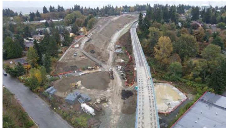
Earthwork along the new SR 509 alignment near Sound Transit's Federal Way Link Extension work zone in SeaTac
